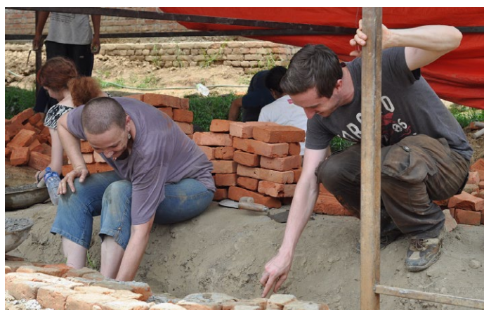
Projects Abroad volunteers lay bricks for the new classrooms at Sunrise School
